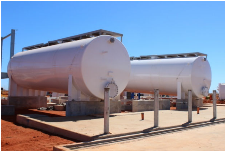
Pilbara Emulsion Plant, Western Australia
