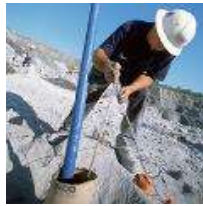
End-of-Hose device patented, allowing all gassing to take place in the borehole
